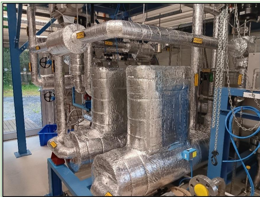
Figure 1: CEEGS facility after commissioning.
